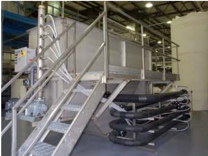
IWWS 200 GPM Phys/Chem System in Kingsport, TN earned an award for Excellence in Wastewater Pretreatment from the city
